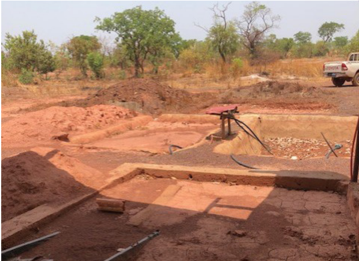
FIGURE C1. A full settling pond in Guinea
